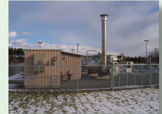
Metering and Regulating Station
